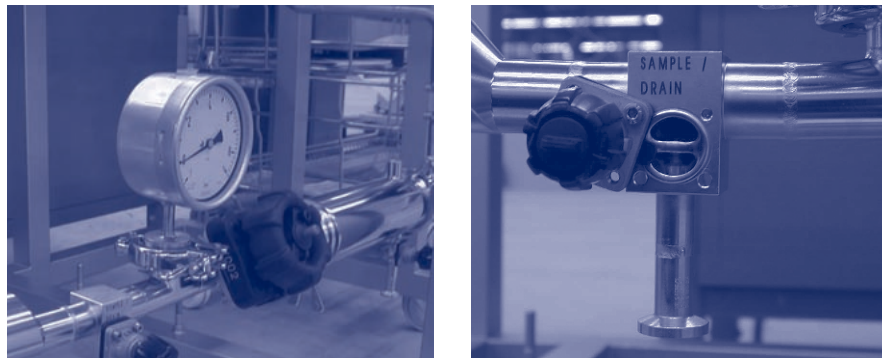
Figure 19: Design of bleed valves installed upstream of filters.
